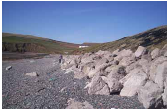
St Bee's beach, Cumbria showing rock armour or rip rap, forming a type of sea wall.
